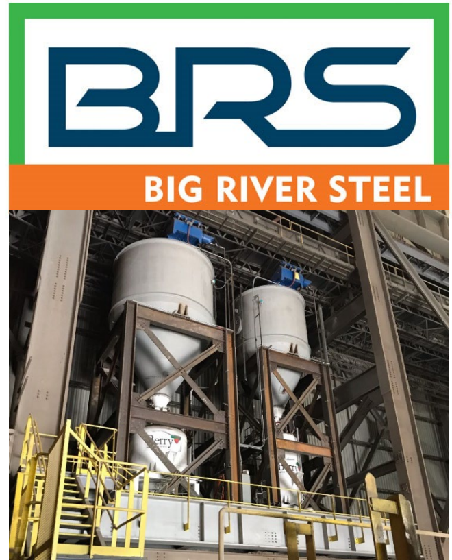
The Berry Metal high efficiency, high volume pneumatic lime injection system was recently commissioned at BRS.
